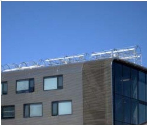
These helical Aerotecture turbines on a building in Chicago have been operating only sporadically.
